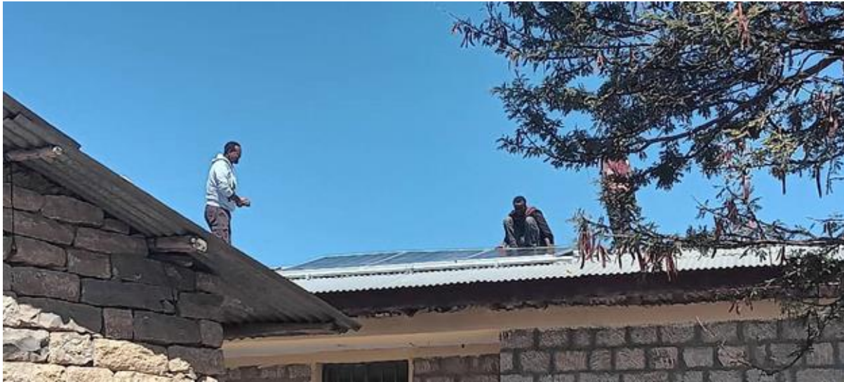
Figure 10: Installed Solar PV at Mitslal Afras Health Post
