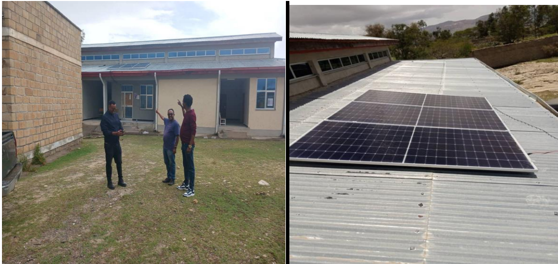
Figure 5: Installed Solar PV at Agazi Health Center
