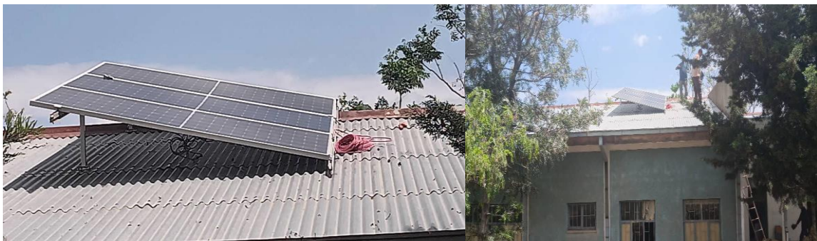
Figure 7: Installed Solar PV at Daerere Health Center
