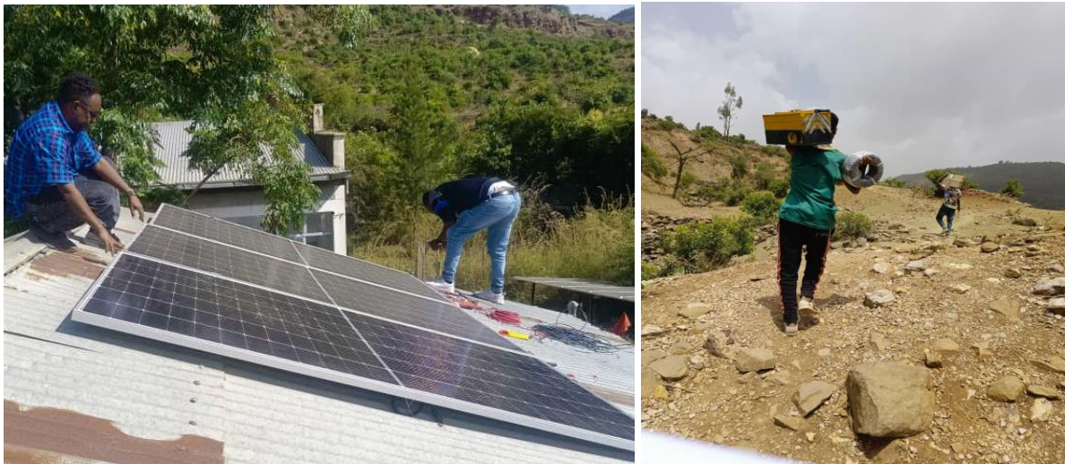
Figure 8: Installed Solar PV at KeretsMay Health Center
