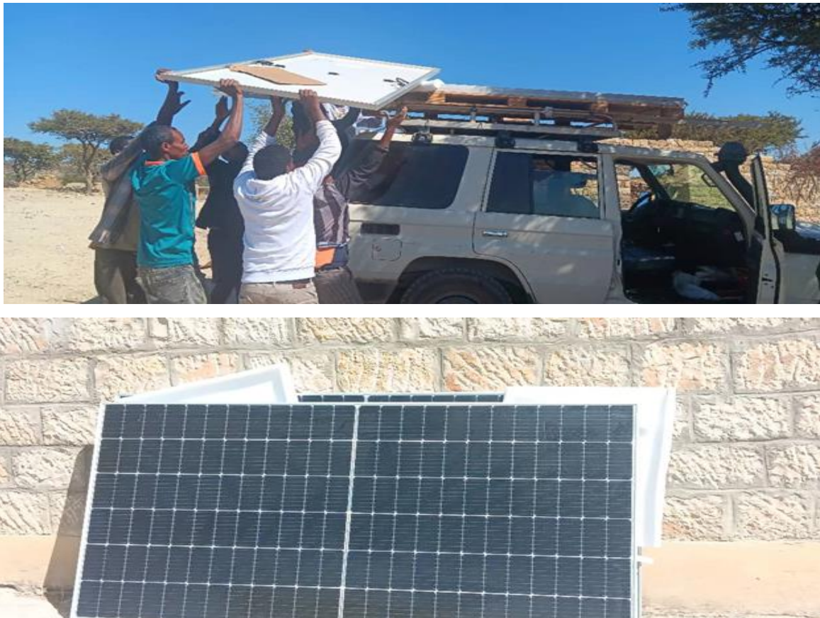
Figure 9: PV Components for Installation-Mitslal Afras Health Post
